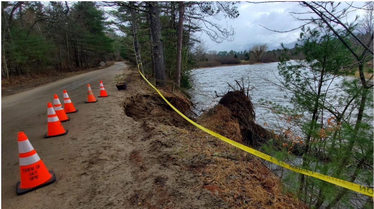
Figure 1: Collapsed tree along River Road looking upstream along West Branch Ausable River during flooding in April 2024.
